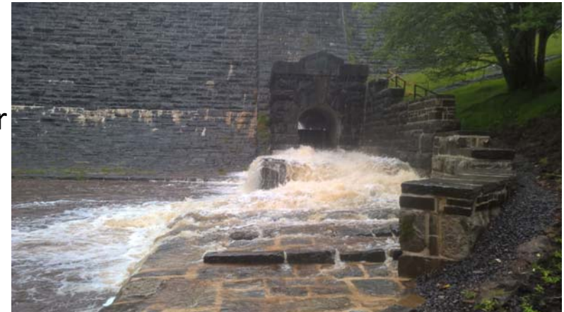
Outlet culvert in operation
